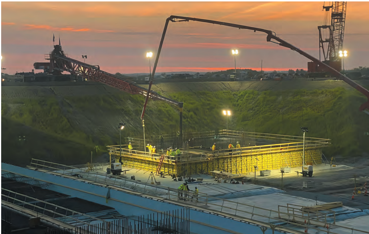
Intel's Ohio One construction teams began the concrete pour in May of this year.
